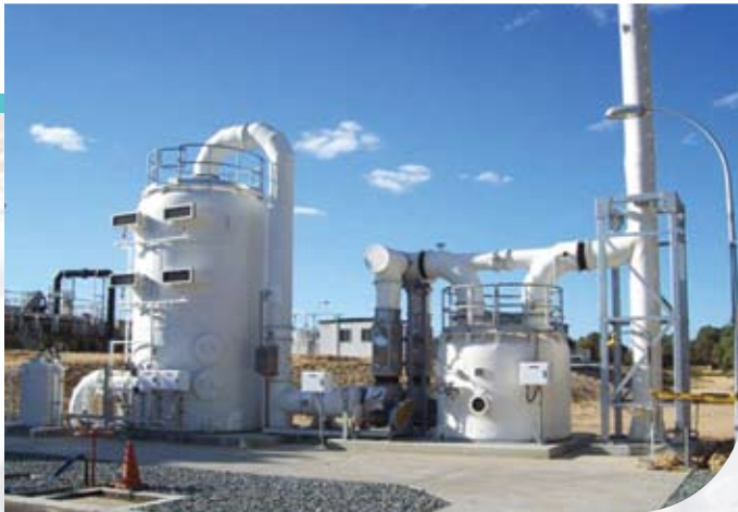
Halls Head WWTP, Australia
