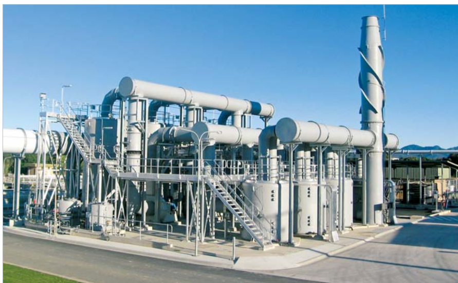
Merrimac WWTP Odour Control Facility.
