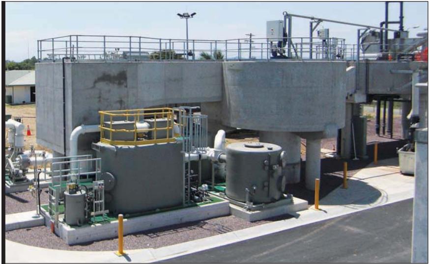
The odour control facility at the Mackay South recycling works.
